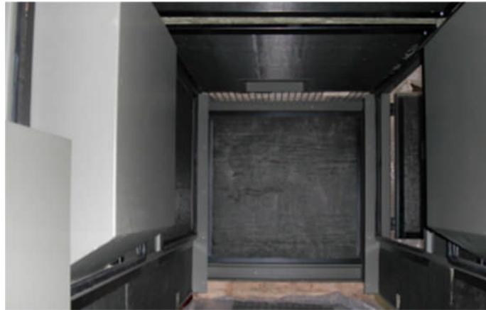
Picture 3-Inside a soundproofed generator set
