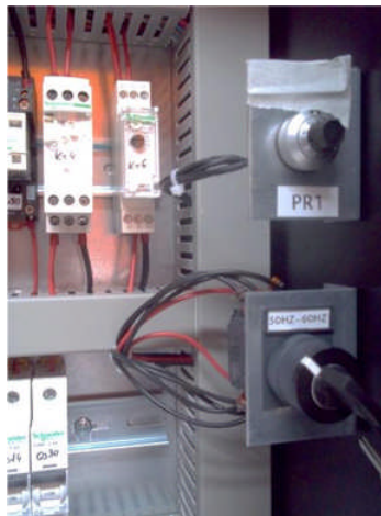
Picture 43: Voltage potentiometer and frequency selector switch
